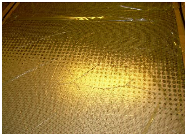
Infusing all bulkheads for both floats in one panel, both sides simultaneously
